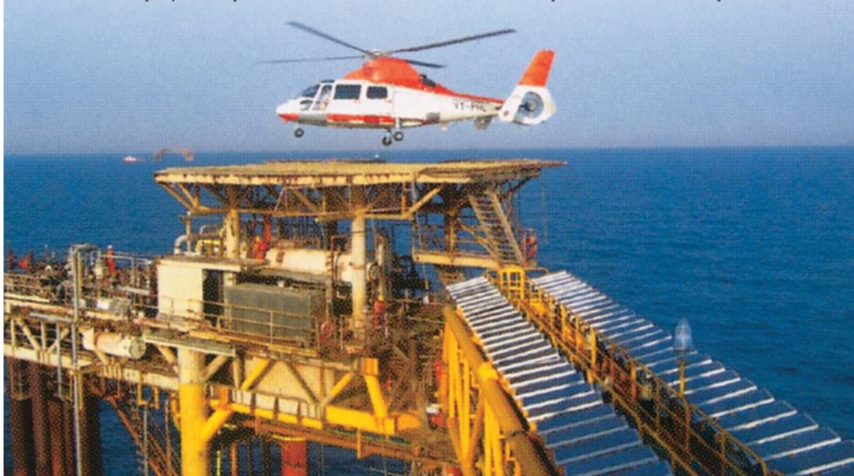
Solar power system for ONGC's offshore platform
