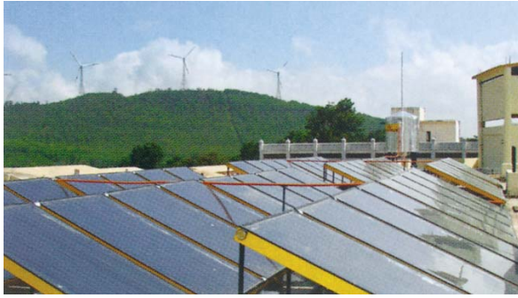
Solar water heating systems at Tirumala, Tirupati temple
